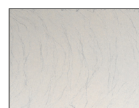
COVERAGE TOO LIGHT
